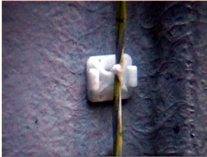
Figure 4.1 The strips pads were affixed to the wall using the supplied double sided tape after cleaning with Kleener Blå
