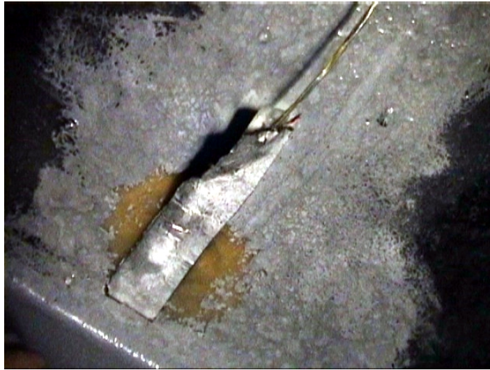
Figure 4.2 Some of the ABM 75 foil covered putty and strips pads fell off under panel 5. This did not affect the measurements, but should be noted in case a long-term measurement is initiated
