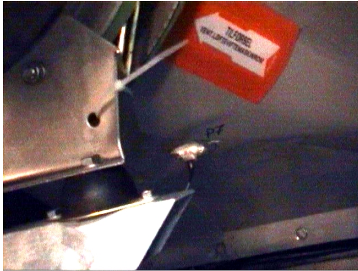
Figure 3.15 Pressure sensor P7 was mounted in a Teflon holder. The holder was inserted in a 16 mm diameter hole in the air inlet and fixed using Sikaflex
